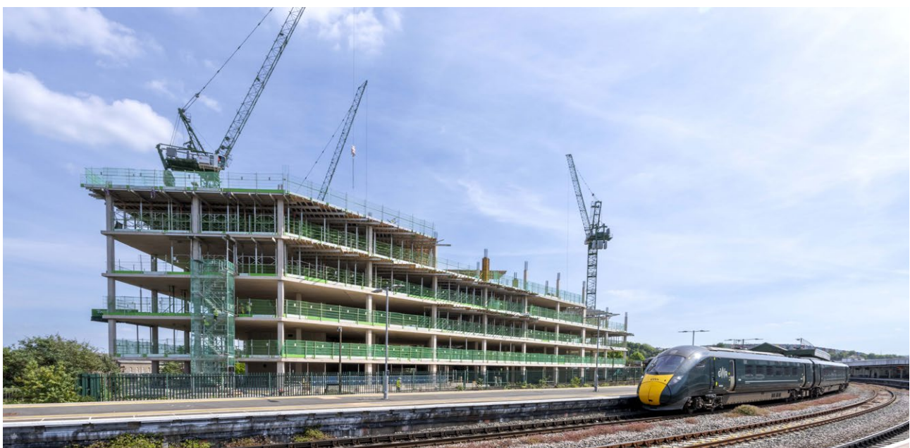
A collaborative approach was instrumental to emissions reduction on the TQA1 building in Bristol.
