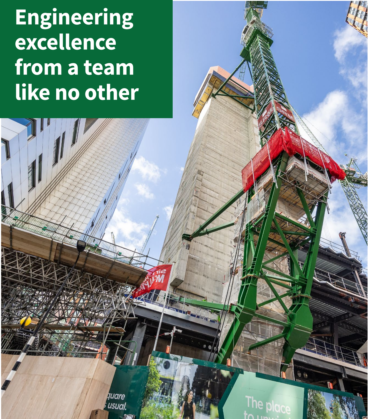
The eye-catching tower crane arrangement at 2 Finsbury Avenue matches ingenuity with technical know-how.
