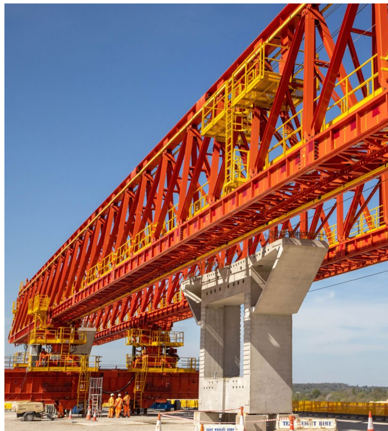
A colossal exercise in civil engineering, the viaduct is as complex in construction as it is elegant in design.
