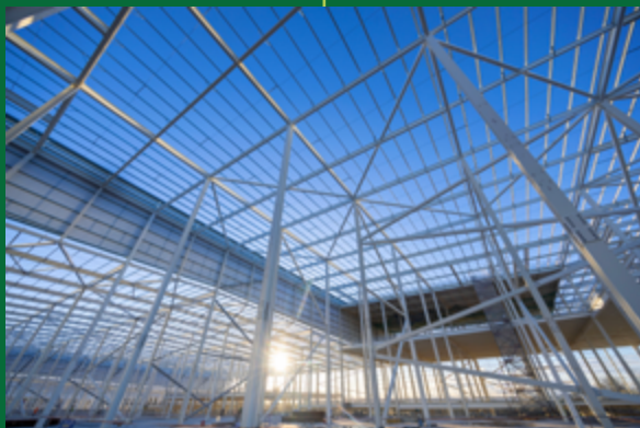
We completed construction of the steel frame of the Agratas battery plant in Somerset.
