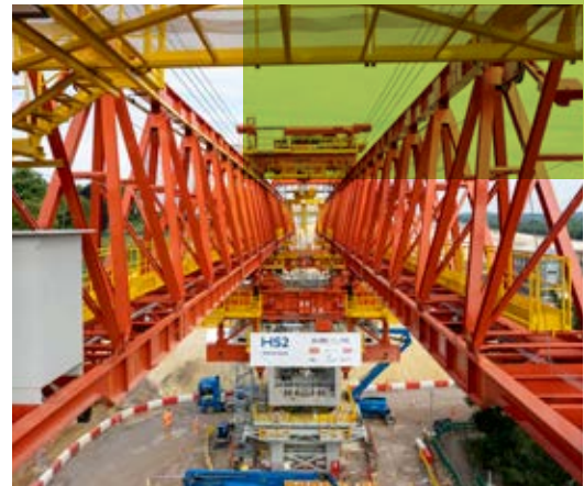
In May 2022 the launching girder that will assemble the Colne Valley Viaduct installed the first of the 1,000 segments that will support the bridge. The 160m long girder is 18m high, 18m wide and weighs in at around 700 tonnes.
