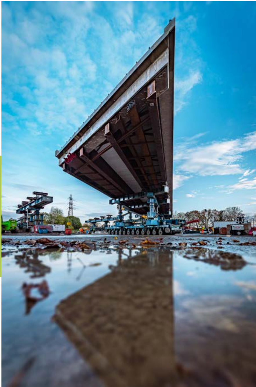
The 67m steel structure for the A533 Expressway bridge was built off-site at a compound close to the M56.
