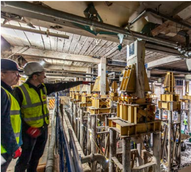
At the Westbury Hotel in Mayfair, highly technical basement works have required close collaboration with Transport for London.
