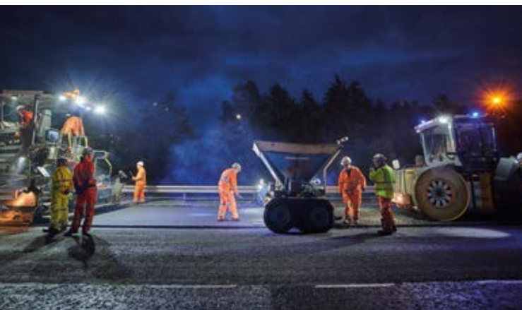
Capital Ventures operates the 30 year concession responsible for this network of strategic dual carriageways. Initial upgrading of the network including refurbishing bridges and viaducts has been followed by ongoing responsibility for routine operations and maintenance of the network.
