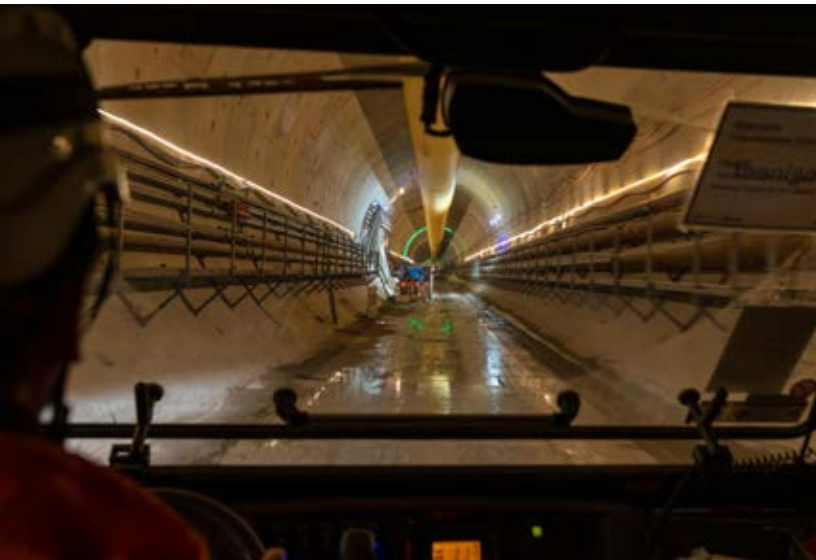
Tunnel Boring Machine (TBM) Florence completes her first mile. Florence and her identical sister TBM 'Cecilia' are excavating twin ten mile long tunnels. They are self-contained underground factories; digging the tunnel, lining it with concrete wall segments and grouting them into place as they move forward.
