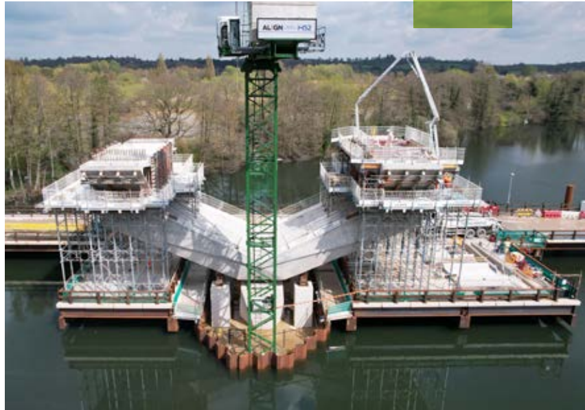
Our team has supplied 11 tower cranes to the Align JV which is working on the Colne Valley Viaduct as part of the HS2 Civils Package C1.
