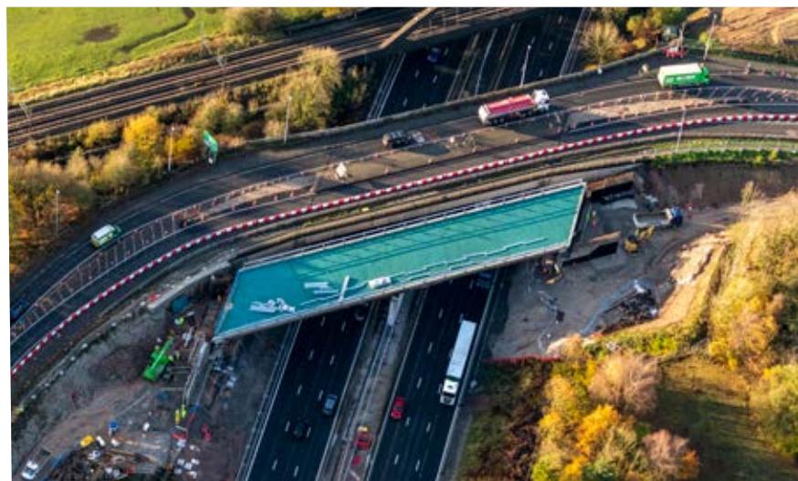
The A533 Expressway bridge project included the off-site construction of a new 67m span steel bridge and its transport along the motorway to be installed.
